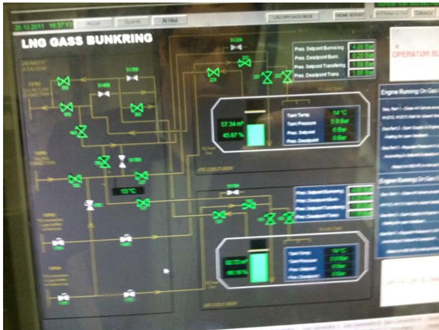
Bunkering control screen
