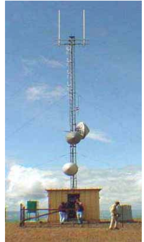
Southwest Region Haystack Butte Wireless Site
