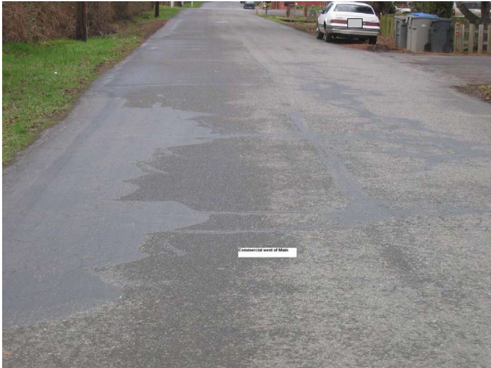
Pavement Condition 52 (Poor): Commercial Street west of Main and 99W Overpass
