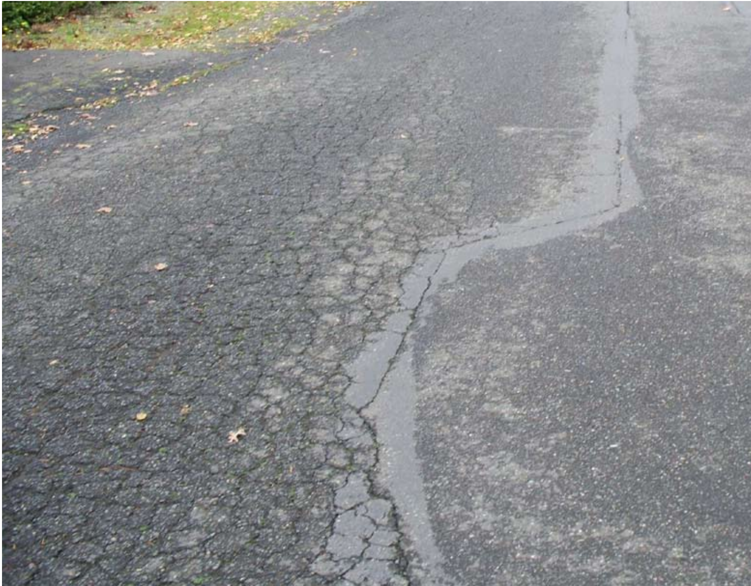
Pavement Condition 20 (Very Poor): Beveland Street 500' east of 72 nd Avenue
