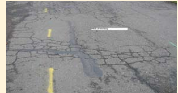
Pavement Condition 34 (Very Poor)
