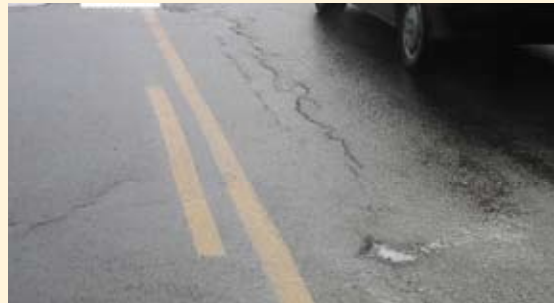
Pavement Condition 64 (Fair)
