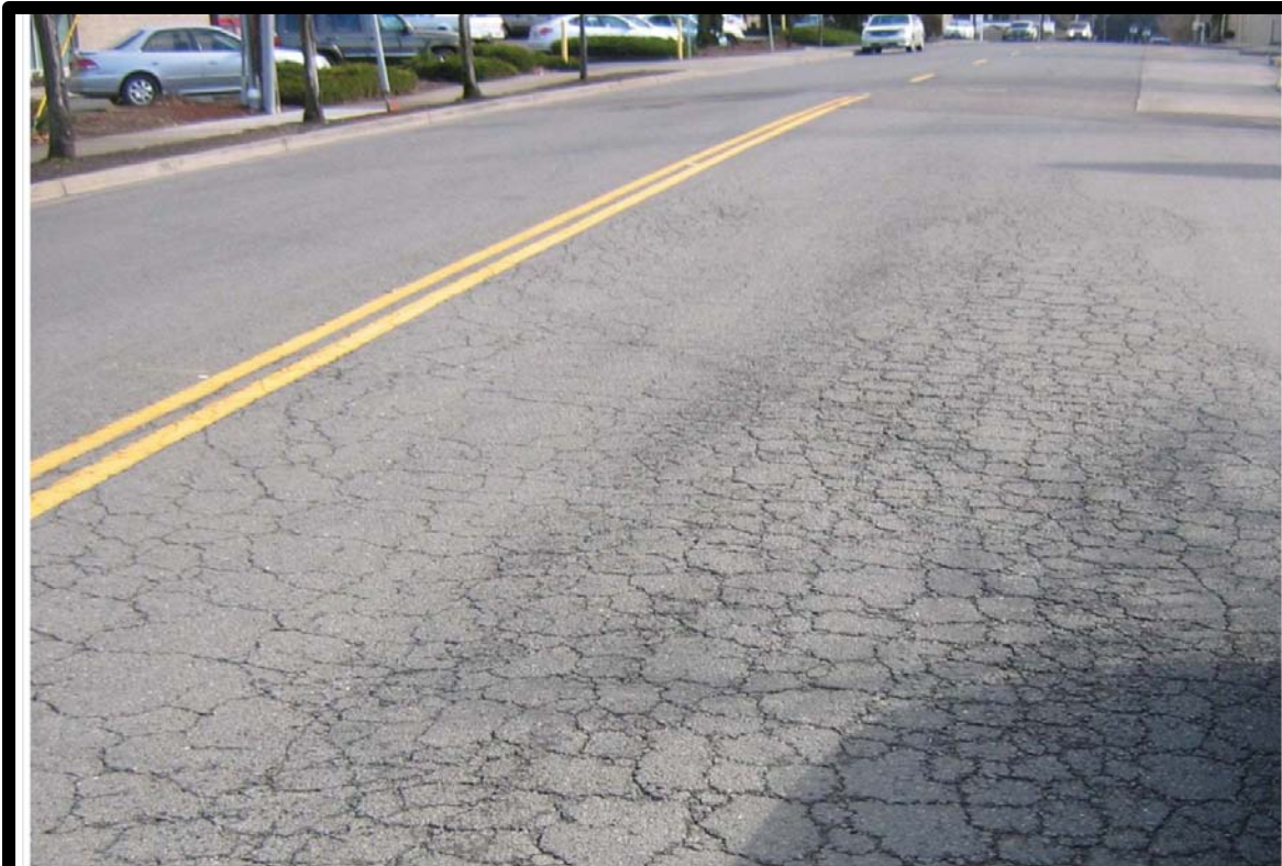
Pavement Condition 42 (Poor): Commercial Street east of Main Street
