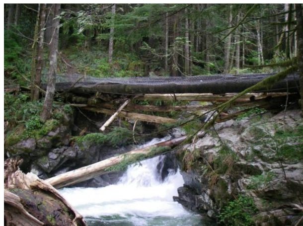
User-built structures such as this log bridge at Reiter Foothills Forest with chicken wire nailed to the top present risks to public safety and potential liability issues for DNR.
