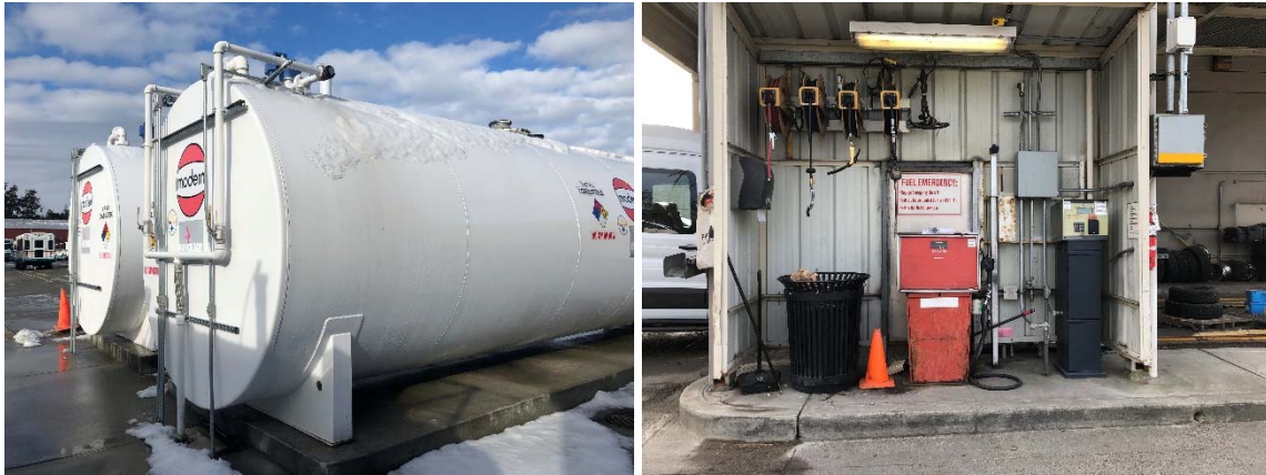
Left to right: Fuel tanks at Island Transit's Coupeville base; fuel pump at King County Metro's Atlantic/Central base.
