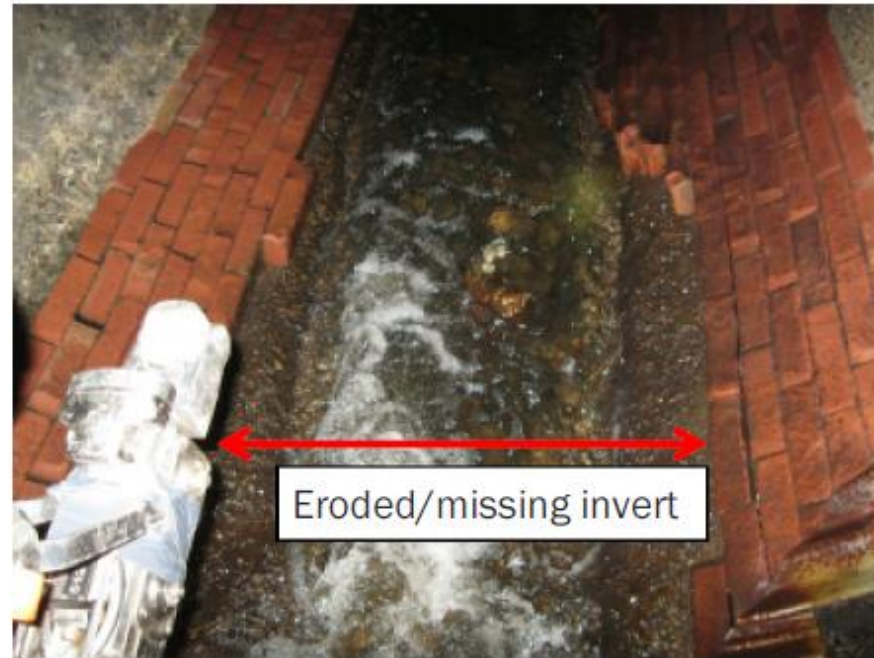
Figure 2-3. Ellipse: missing invert (170')
