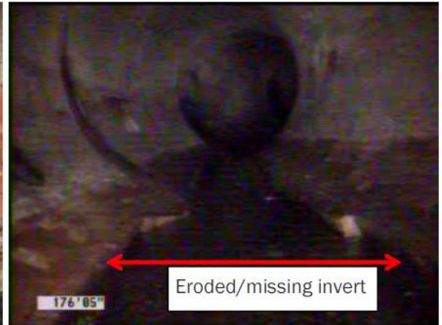
Figure 2-4. Ellipse: missing invert (176')
