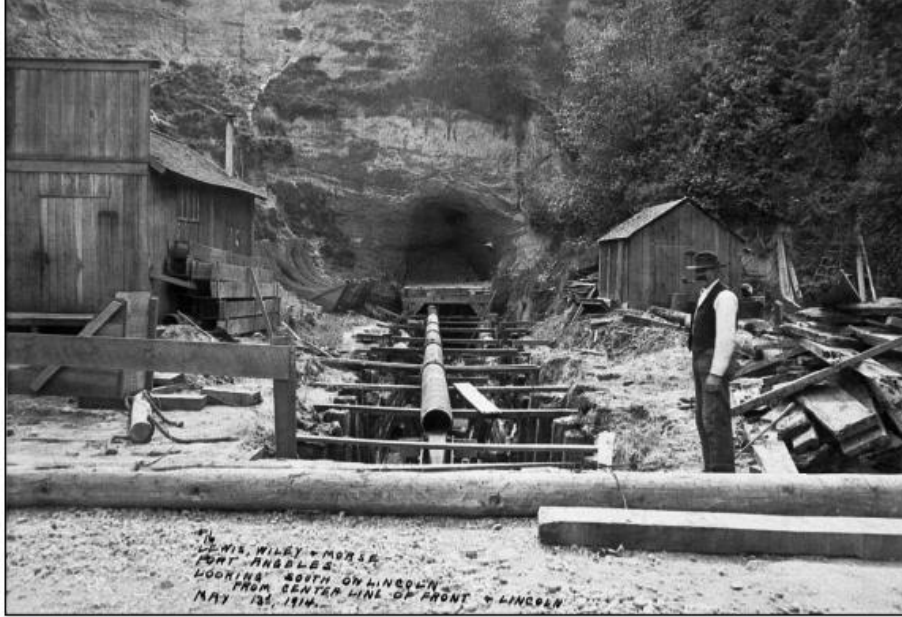
Picture 8: Construction of culvert north at intersection of Front and Lincoln (looking south)
