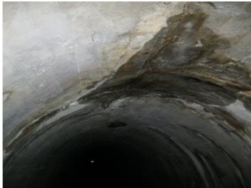
Figure 2-9. Ellipse: crack with infiltration (335')
