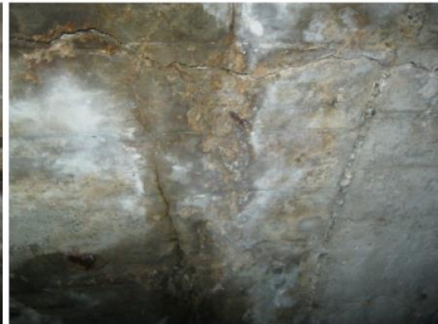
Figure 2-10. Ellipse: crack with infiltration
