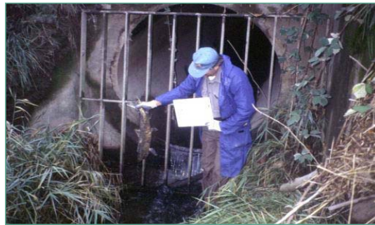
Trash Racks and Flap Gates
