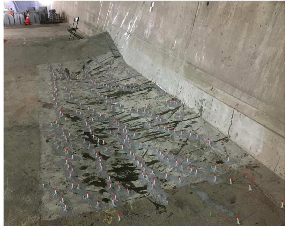
Small “syringes” are placed into affected areas and used to channel epoxy into the cracks.
