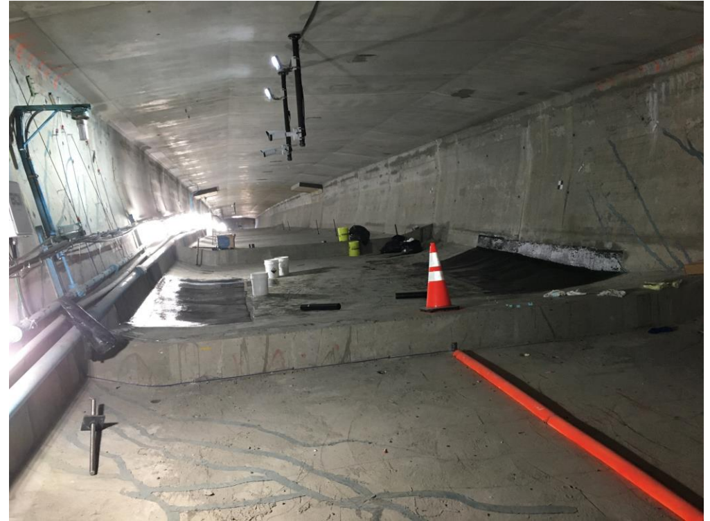
Epoxy crack injection and carbon fiber wrap in a section where many of the larger cracks were identified.
