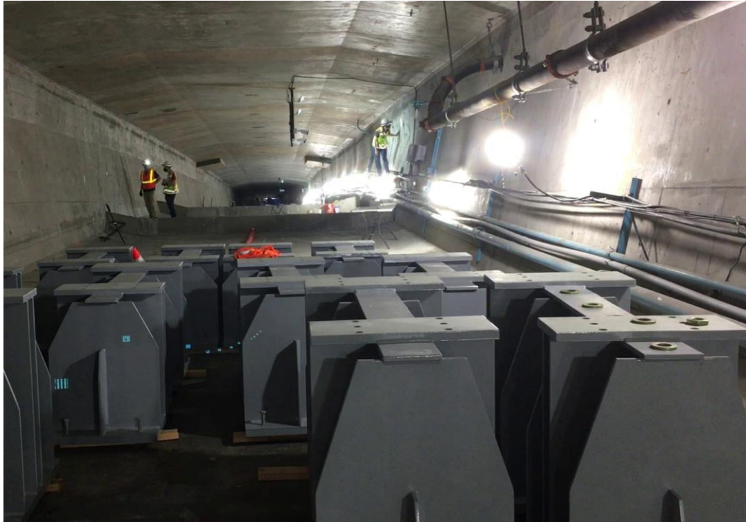
Crews working inside the bridge. In front, the post-tensioning brackets used to reinforce the concrete.
