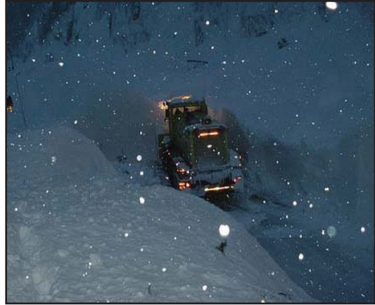
Crews worked all night to clear a snow slide 30 feet deep
