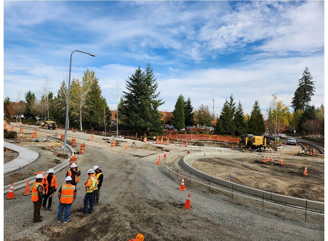
Crews plan the next steps of the Redmond Ridge roundabout at NE Alder Crest Dr.
