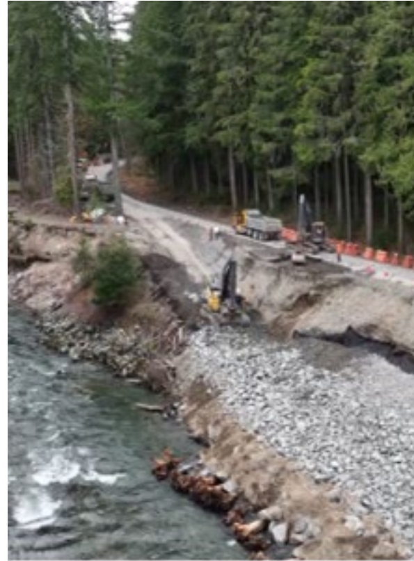
Marten Creek Culvert Unexpected flooding damages culverts and infrastructure
